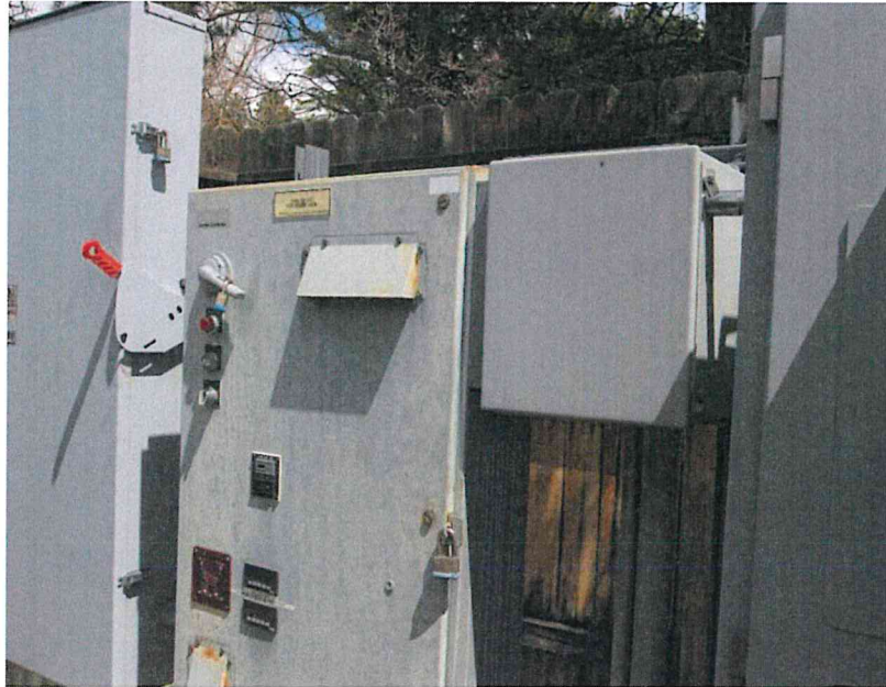
Figure 3: Existing Electrical Equipment Line Up
